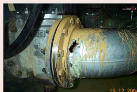
Corroded pipe spool from high acid leach tank
