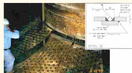
Catalyst bed failure
