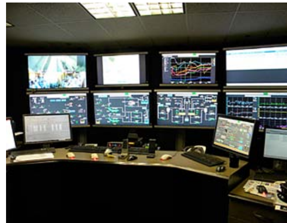
Wash Plant Control Room
